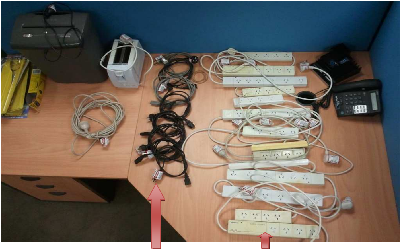
Failed Office appliances – Damaged computer power leads and power boards under desks
