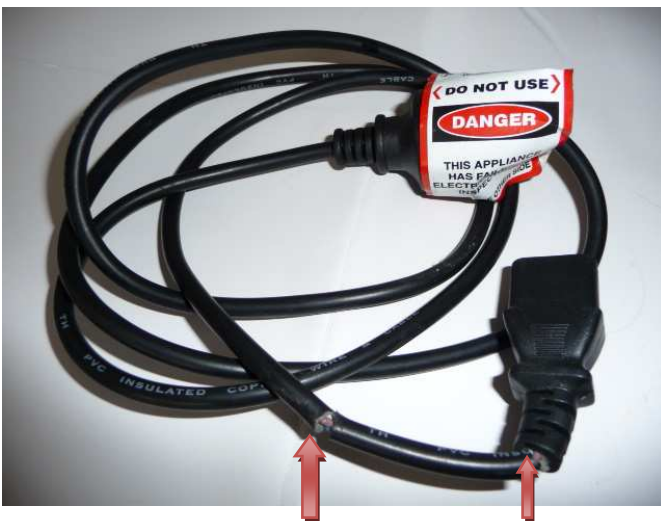
Computer Power lead with cuts in the black outer insulation
