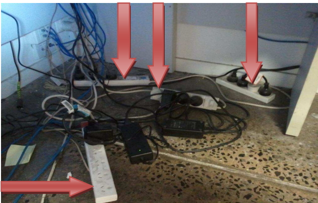
Four power boards plugged into a double power point
