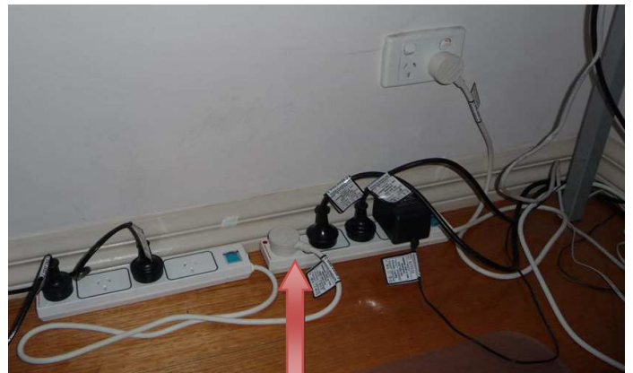
A second power board plugged into the first one – overload?
