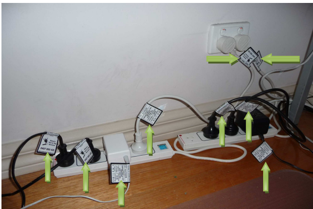
Arrow's show the tags installed after successful testing
