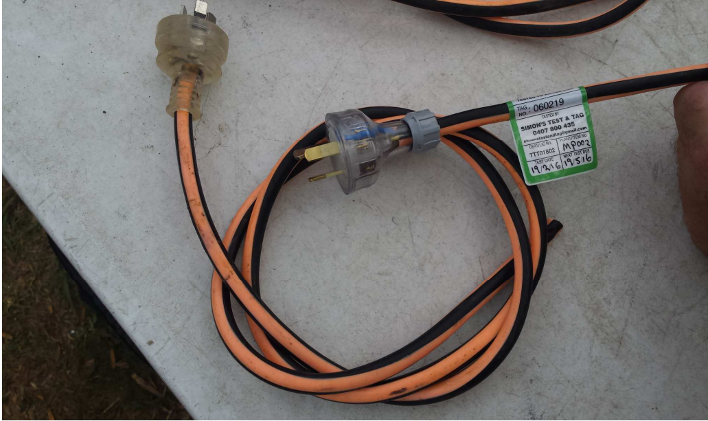
* Appliance MP002 Passed a re-test after a new plug was fitted to the damaged lead
